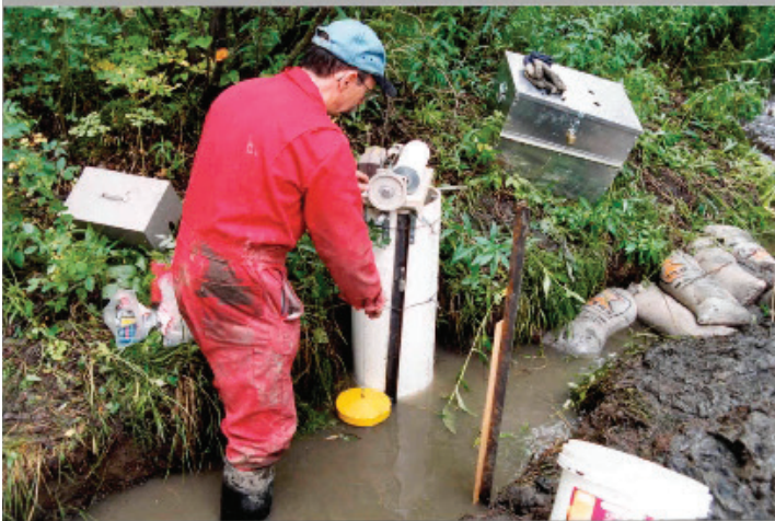
Figure 4.15e. Still well installation August 2000.
