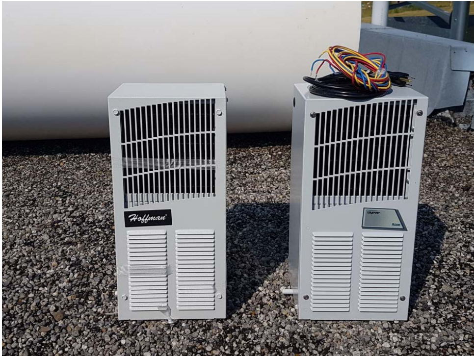
Figure 2. Replacement of temperature control unit during annual LiSAmobile maintenance conducted by an Ellegi engineer.
