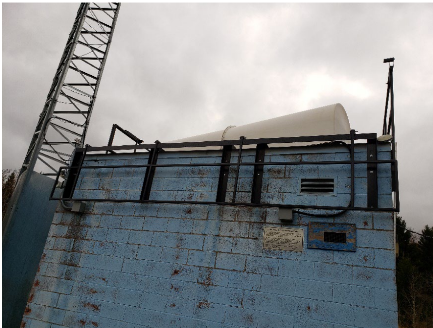
Figure 5. Front hand railing in the open position at the Bellevue pump house (Turtle Mountain, Alberta) so the railing does not interfere with LiSAMobile readings.
