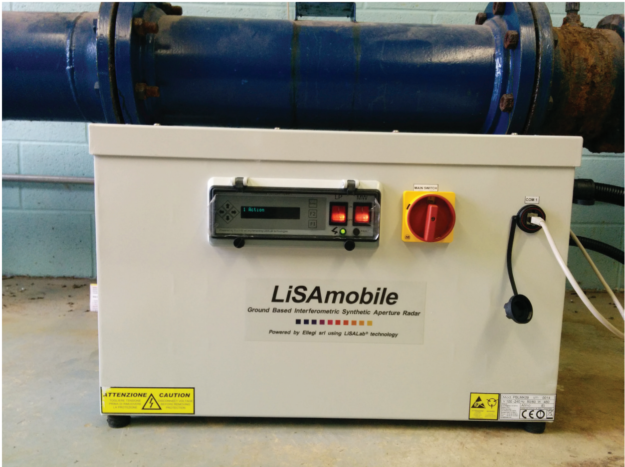
Figure 5. Power box located inside the pump house building and connected to the LiSAmobile system on the pump house roof.
