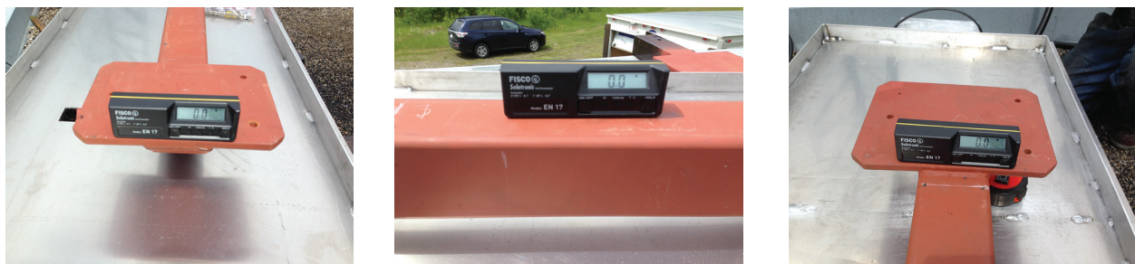
Figure 6. Pedestal installation for optimal trajectory angle of LiSAMobile radar head (photos courtesy of Ellegi).
