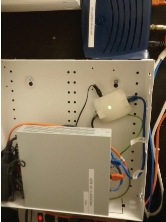
Figure 3. CheckPoint Software Technologies Ltd. Internet gateway, installed at the Blairmore Provincial Building in May 2014.
