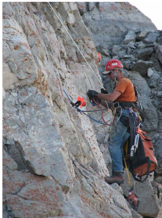
Figure 4. Installation of one of the sixteen prisms on the eastern face of Turtle Mountain during July 2007.
