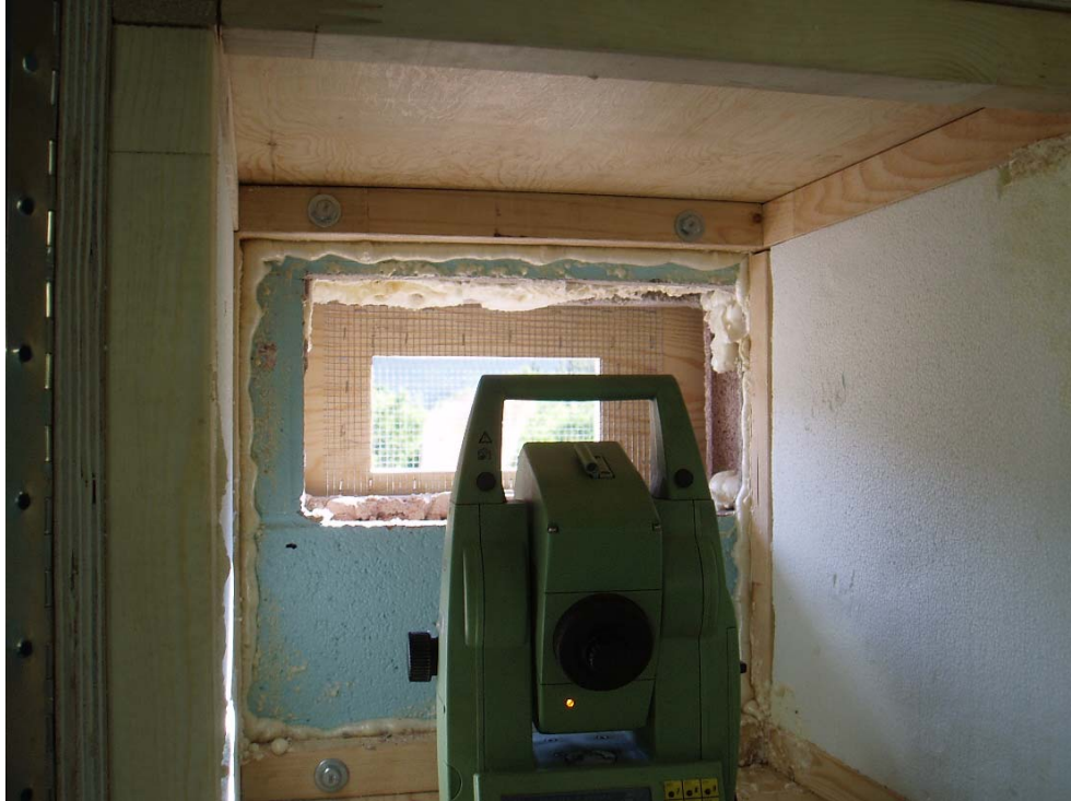
Figure 5. The Leica ‘total station’ installation in the municipal pumphouse at Bellevue, near the base of Turtle Mountain. The total station is in an insulated box and located approximately 3 km from the prisms on the eastern face of Turtle Mountain. Photo: G. Bjorgan, McElhanney Consulting Services Ltd.).
