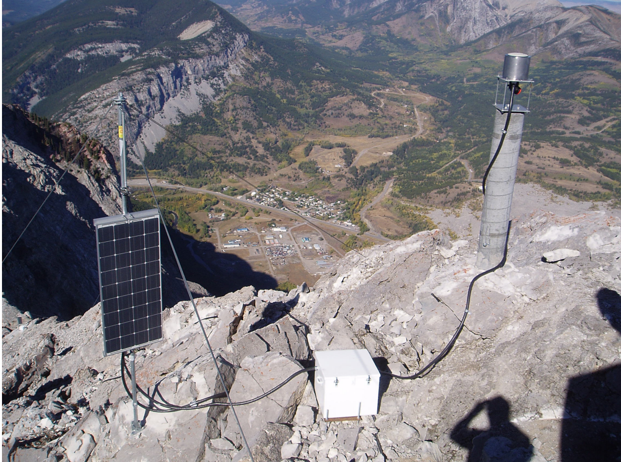
Figure 3. Typical dGPS installation showing concrete pillar with Novatel antenna (right), battery box (centre) and solar panel (left) (Photo: Glen Bjorgan, McElhanney).
