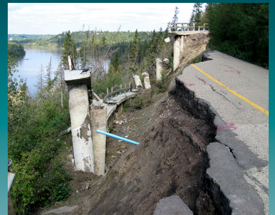
Keillor Road landslide along the North Saskatchewan River in Edmonton, Alberta.
