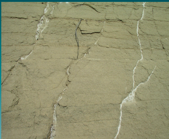
Fractured sand and gravel near Wabamun Lake. Fractures can increase a rock's permeability making it easier for water to flow through the rock. However, sometimes fractures can be filled, effectively sealing them. These fractures appear filled in. Note the white material.
