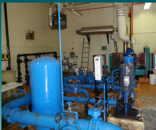
Sophisticated, high-capacity, water-distribution system.
