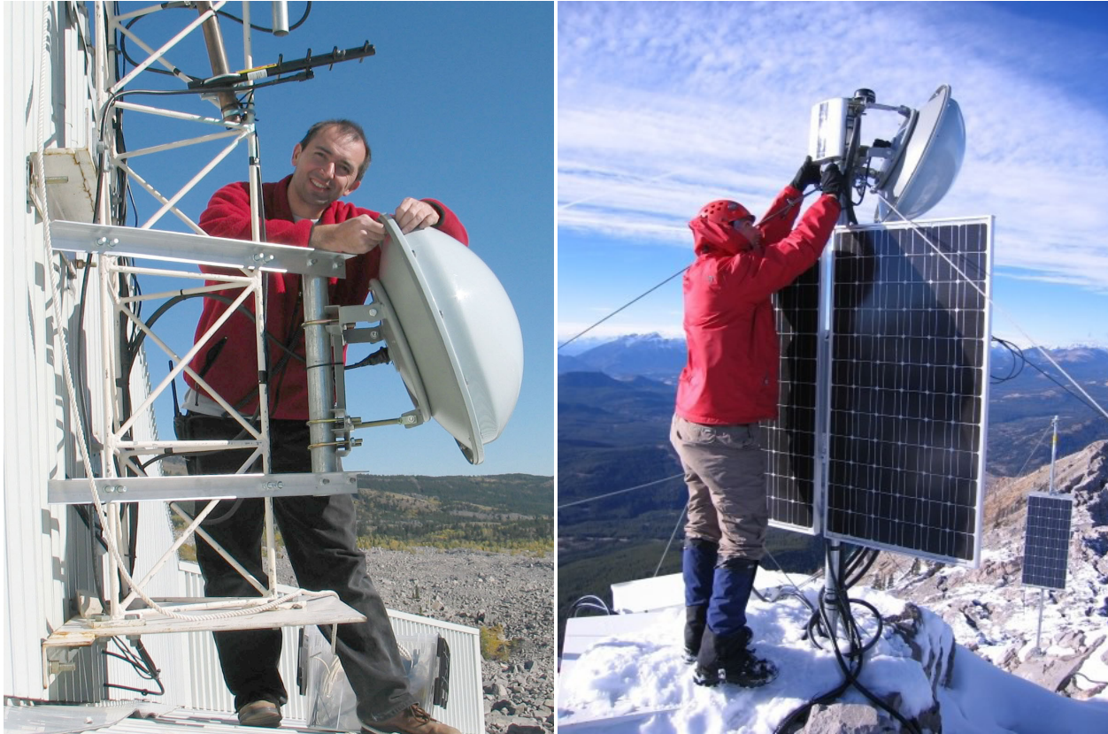
Figure 33. New antennas for the link between the Control Centre at the Frank Slide Interpretive Centre (left) and South Peak station (right), Turtle Mountain.
