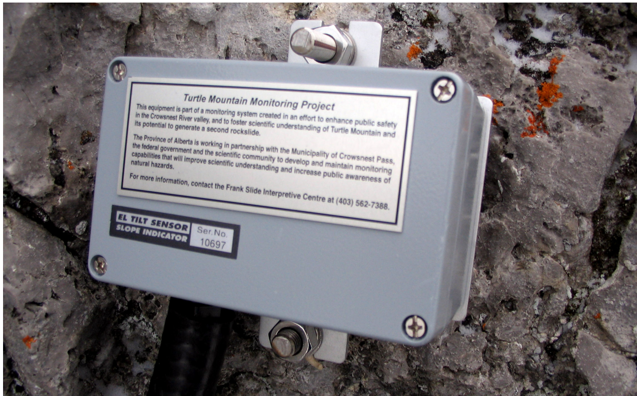
Figure 14. Electrolevel (EL) tiltmeter installed on South Peak of Turtle Mountain. Counter-clockwise rotation of the sensor represents positive tilt.
