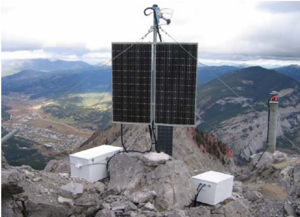
Figure 19. Surface microseismic station installed on South Peak of Turtle Mountain. This station has dual solar panels and battery boxes to accommodate the subsurface microseismic system installed in a borehole drilled nearby.
