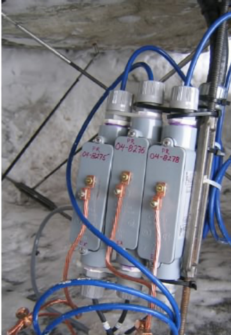
Figure 11. Electrical surge suppressors installed at crackmeter array H on South Peak of Turtle Mountain for protection of instruments from the effects of lightning. Grounding is accomplished by means of the small rock bolt at the lower right.
