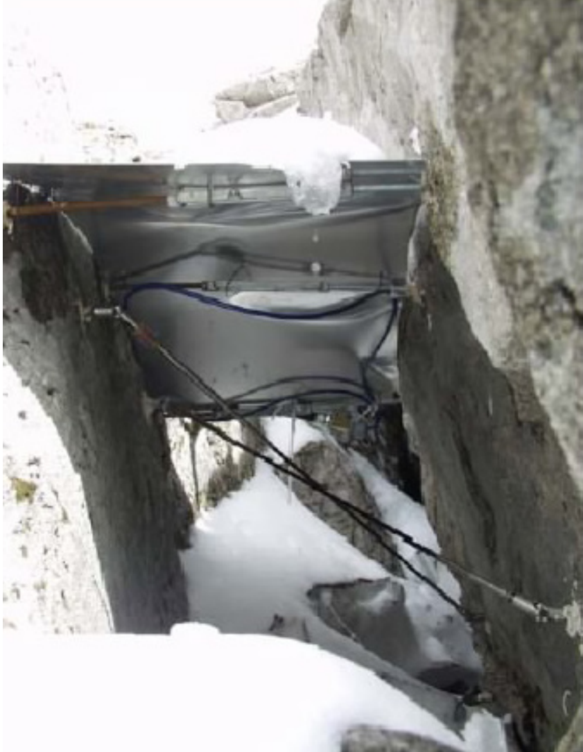
Figure 12. Protective aluminum snow roof installed over a crackmeter array on South Peak of Turtle Mountain to protect it from snow.
